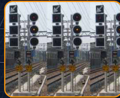
Signalling and Control
