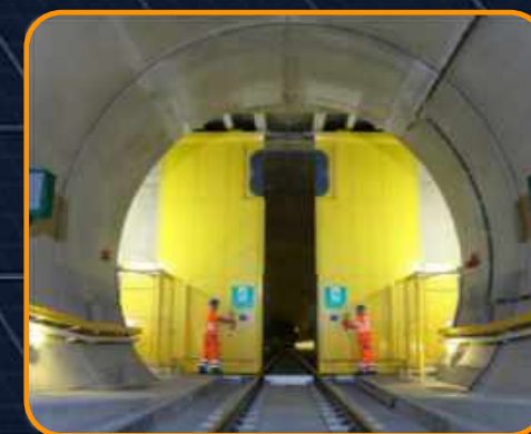
Emergency Doors and Gates
